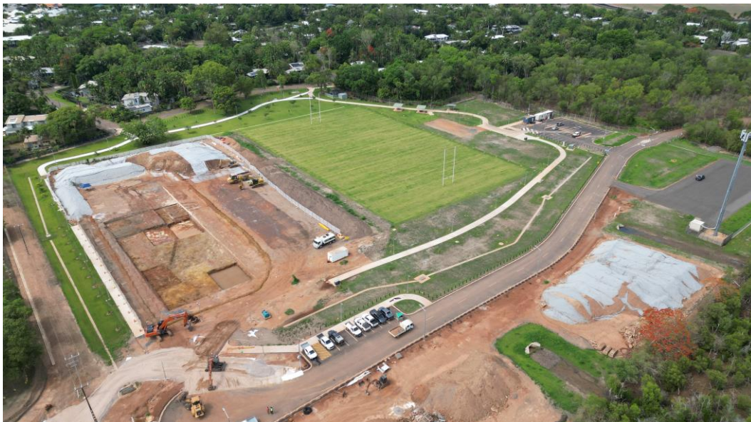
Access extension from Richardson Drive to Ludmilla School and containment cell excavations for asbestosos containing material – Novemeber 2023.
