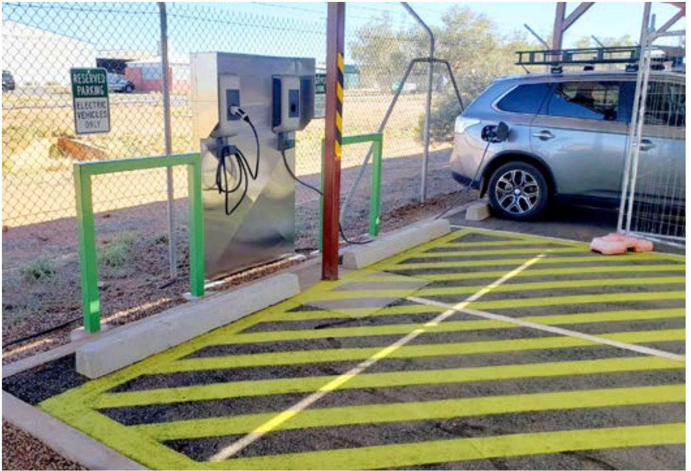
EV Charging station at Alice Springs airport
