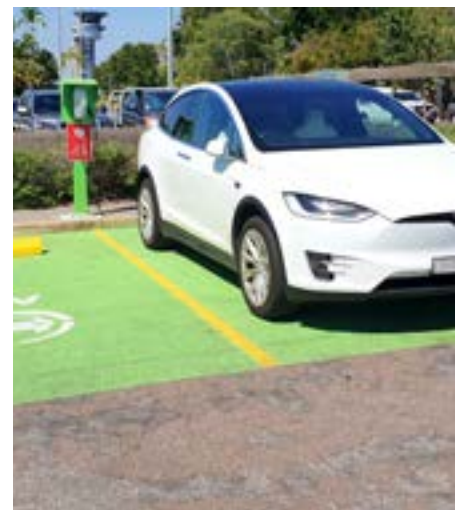
EV Charging station at Darwin Airport
