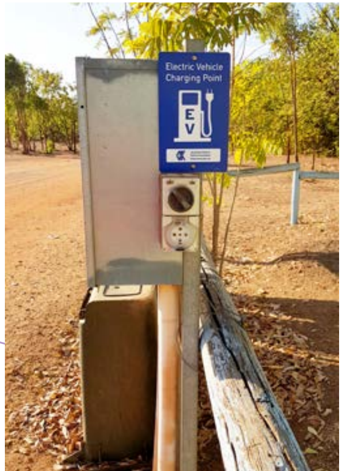
EV Charging point at Mataranka
