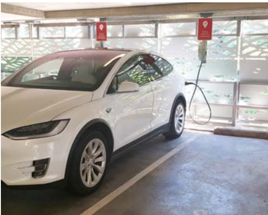
EV Charging station at Darwin Waterfront
