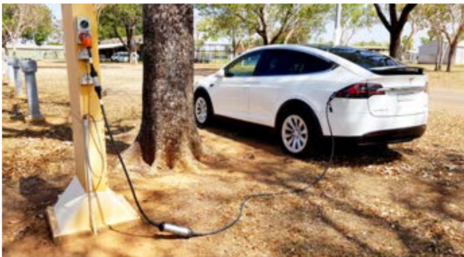
EV Charging point at Katherine
