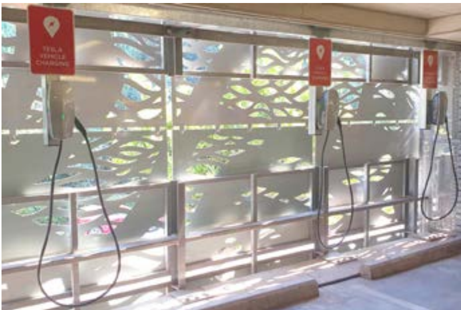
EV Charging station at Darwin Waterfront
