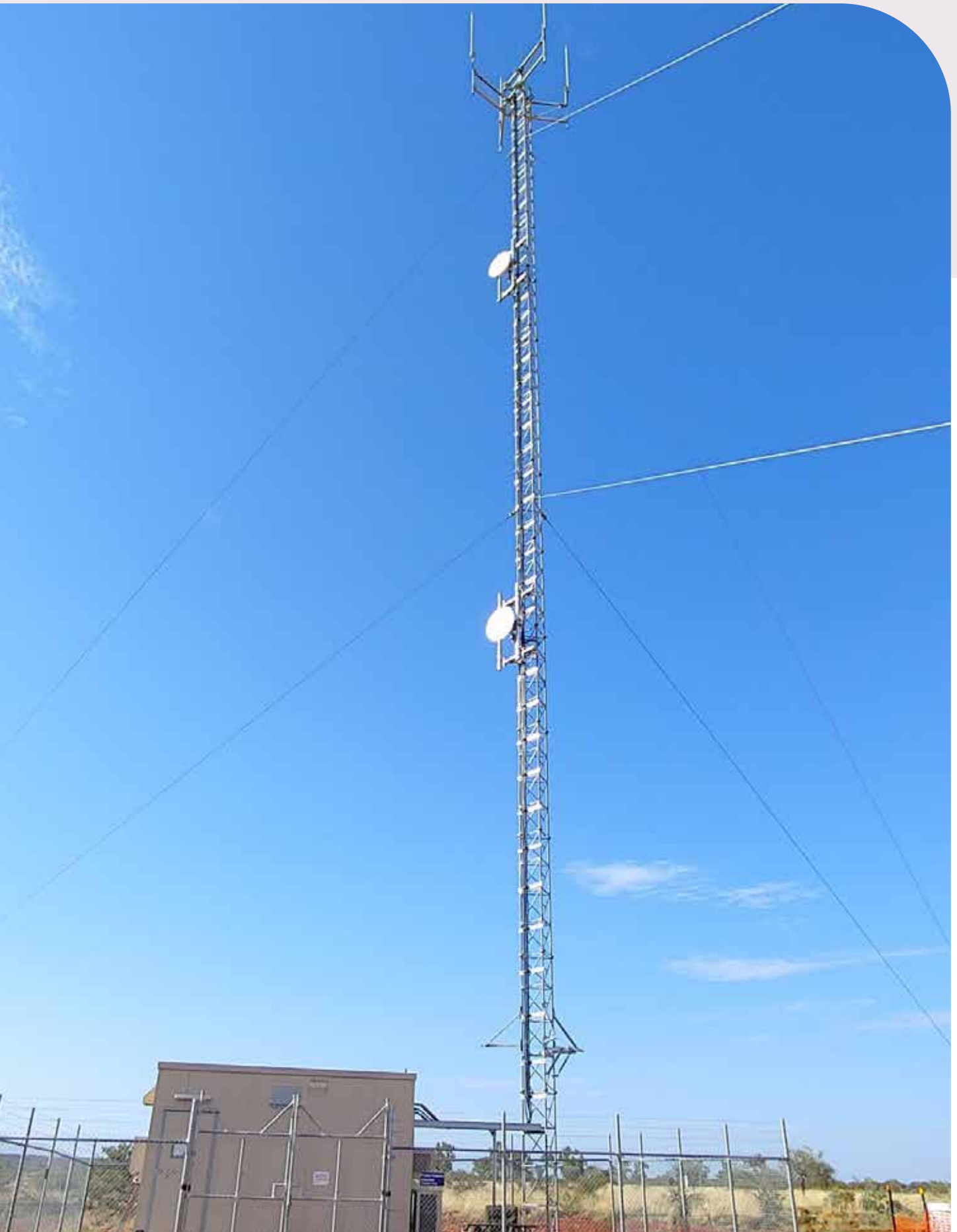
Above: Wutunugurra communications tower. Credit: Telstra.
